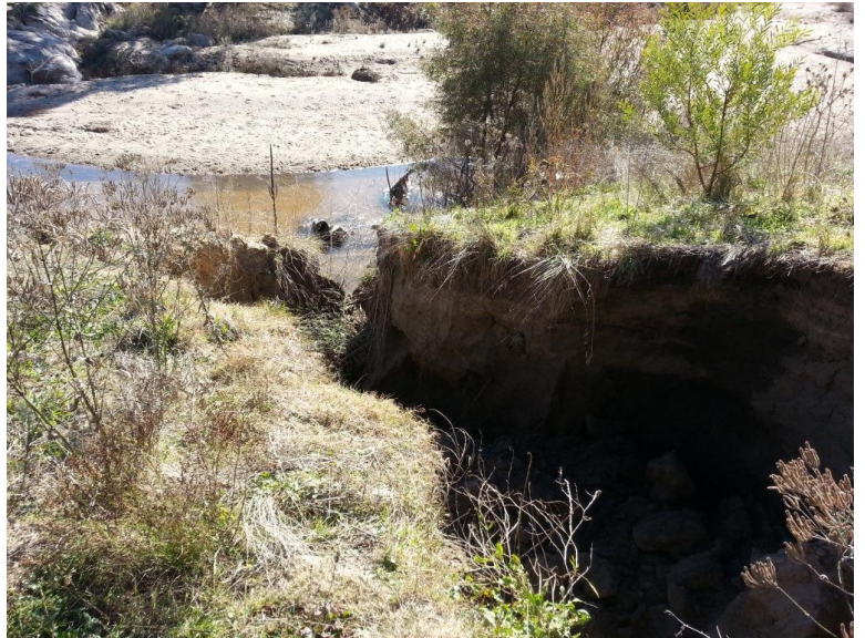
Gudgenby Canyon before erosion control work
